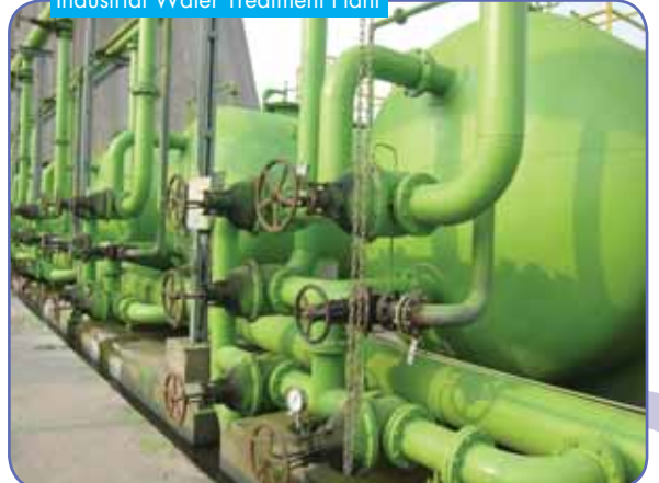
Industrial Water Treatment Plant
